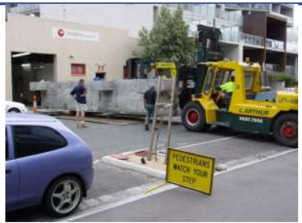
Above: The Relocation of the Rosebank Engineering Ultra-precision Machining Operation was highly complex and needed detailed planning.
